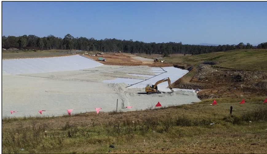
Image 3 – Installation of gravel drainage layer and leachate collection pipework over the protection geotextile
