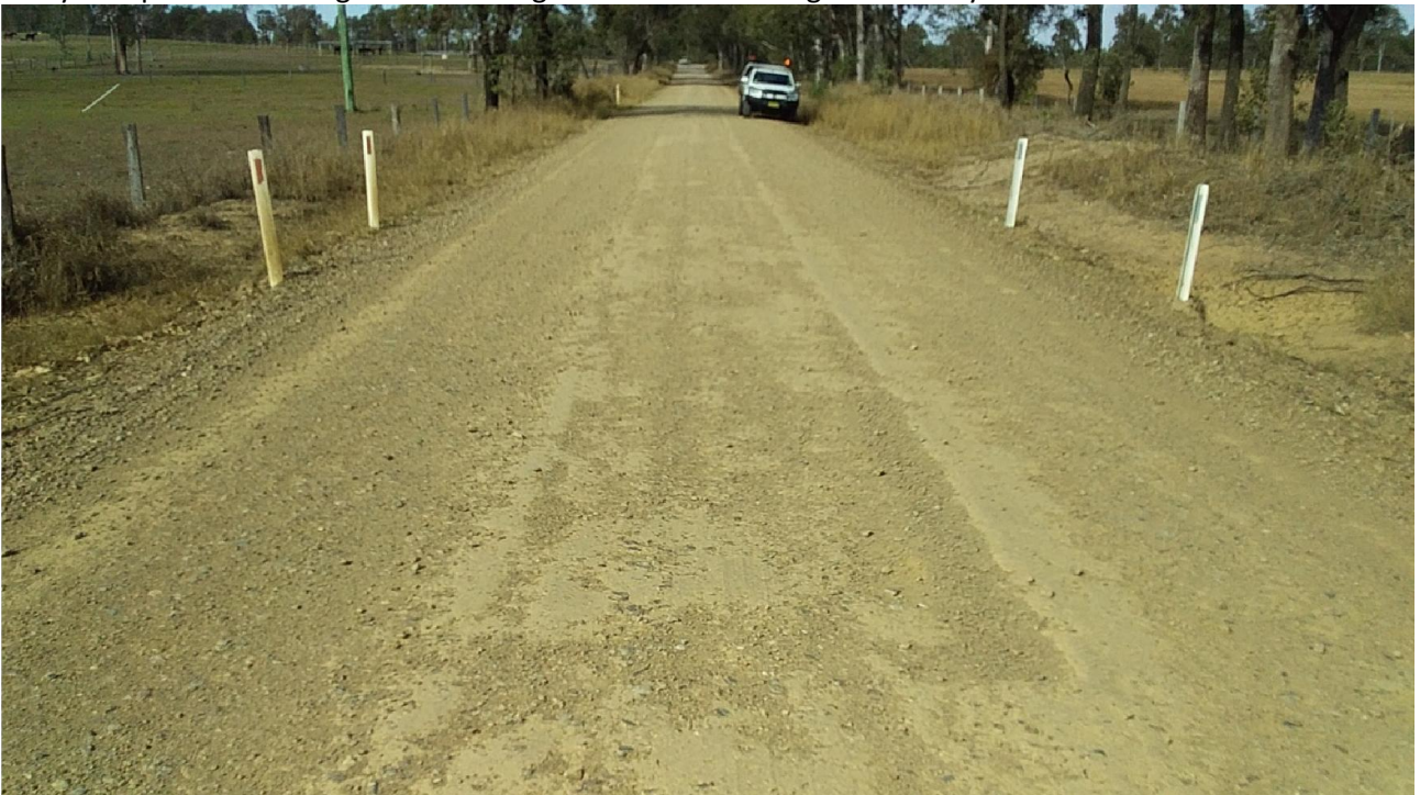
Section 1 Lot 2 Imported Gravel to Specification, excellent shape, minimal stone loss, no effects, no intervention anticipated < 4 months. Has had no major rework, minor pothole repair down centre in isolated locations. That will be 18 months at least and original gravel will still be available for reworking when required.
