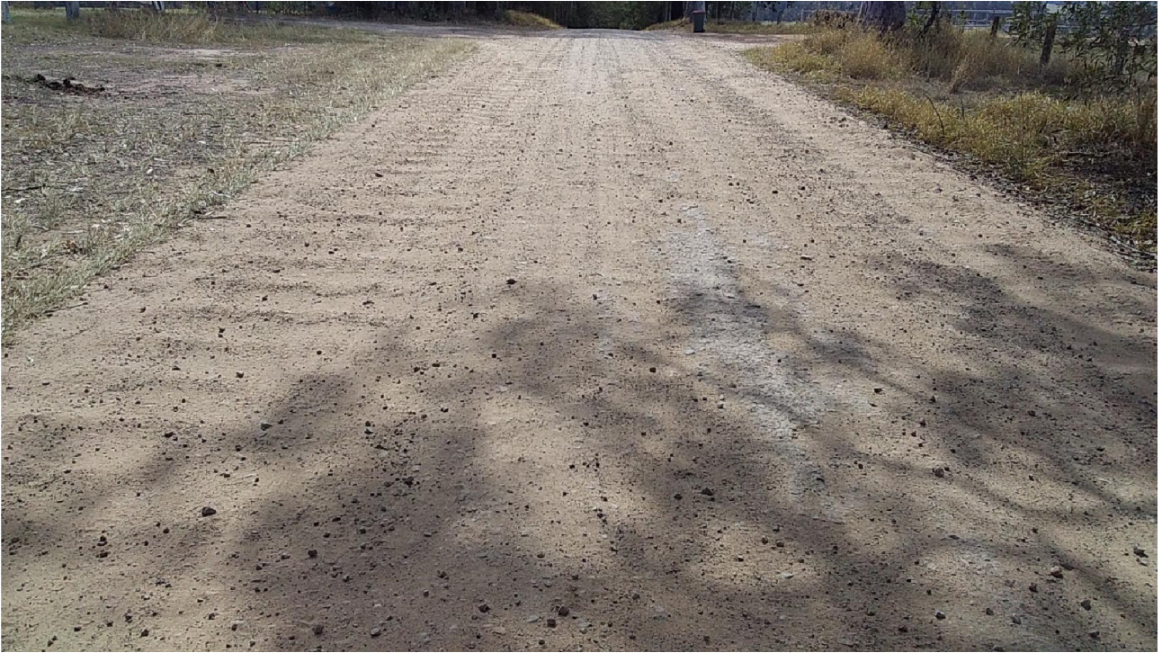
Section 2 Lot 4, Local Gravel with Cement Stabilisation. Has not been reworked, needs rework next grading Cycle, will use exiting material to see how well it reworks.
