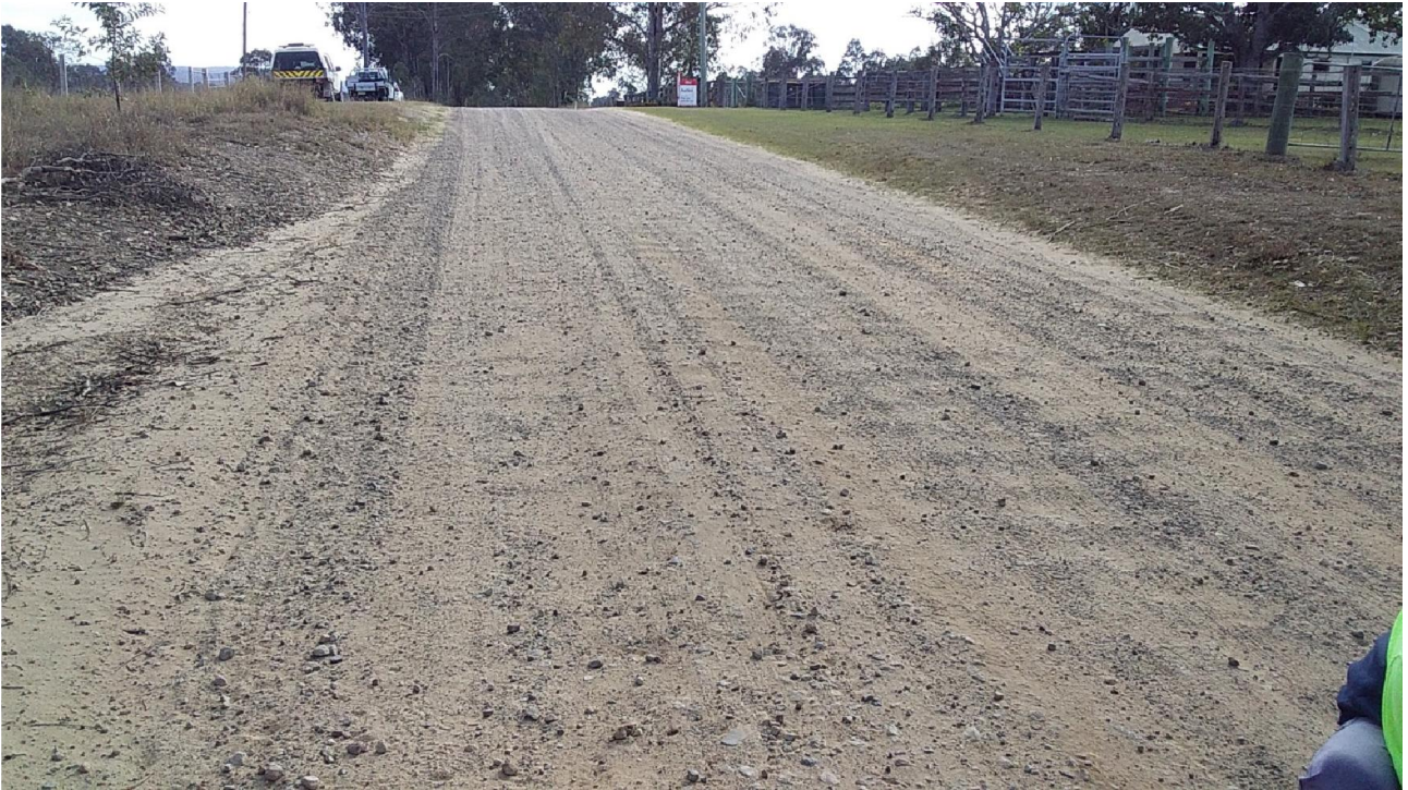
Section 1 Lot 1 Local Gravel, has been reworked at 8 months, flat profile, corrugations, loose gravel, sand, dusty – requires rework again and more gravel as down to original base layer.
