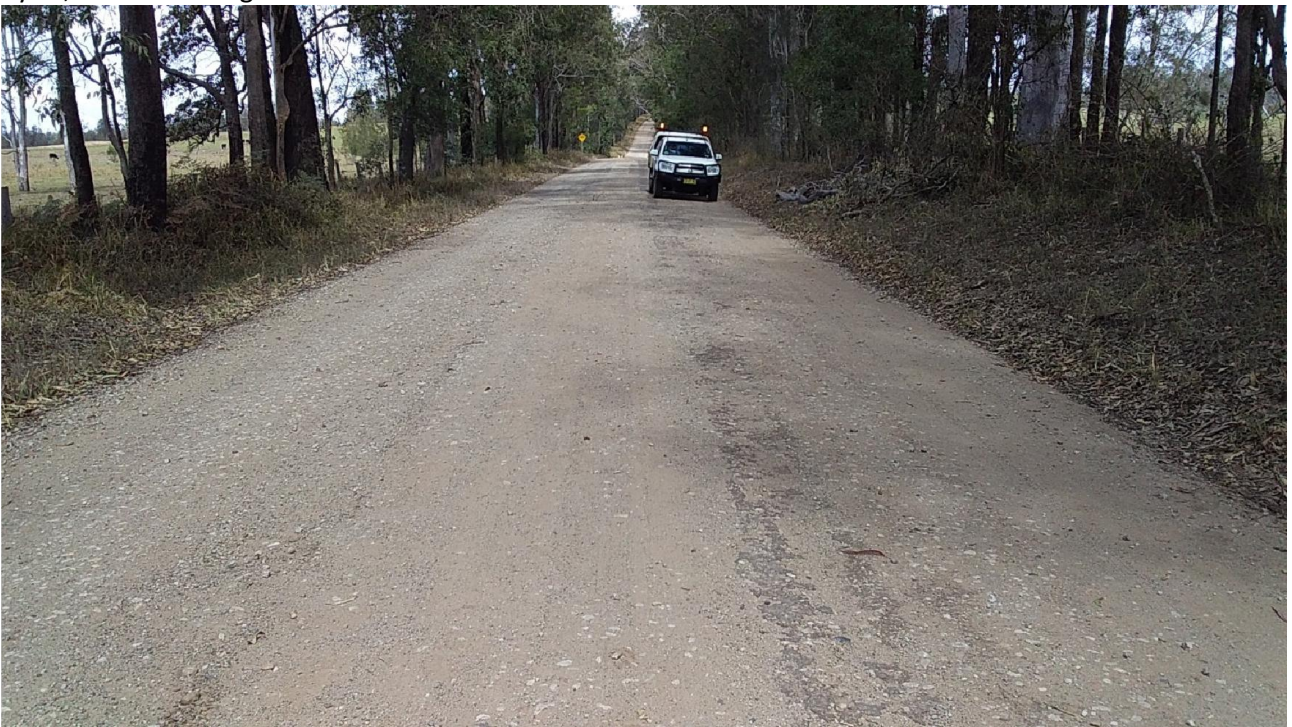
Section 2 Lot 5, Local Gravel with Bitumen emulsion. Has not been reworked and no rework anticipated with 4-6 months. Minor potholes down centre repaired but overall very good condition.
