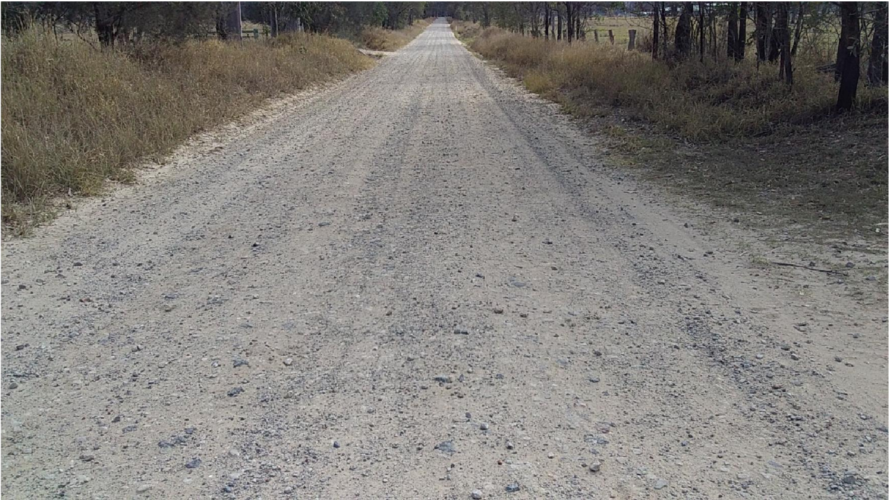
Section 1 Lot 3 Local gravel with PolyCom additive, similar to Lot 1, has been reworked at 8 months and needs rework again with more gravel as down to original base layer.
