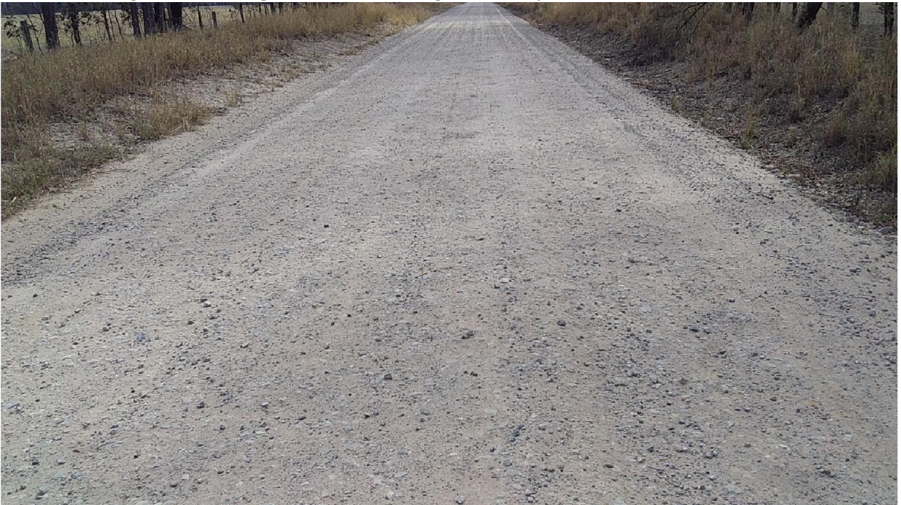
Section 1 Lot 4, Local Gravel with Cement stabilisation, has been reworked after 8 months and has reset reasonably, will not need intervention for another few months at minimum, will monitor.
