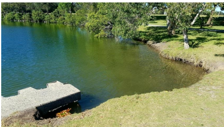
Figure 3: Extent of erosion – southern side
