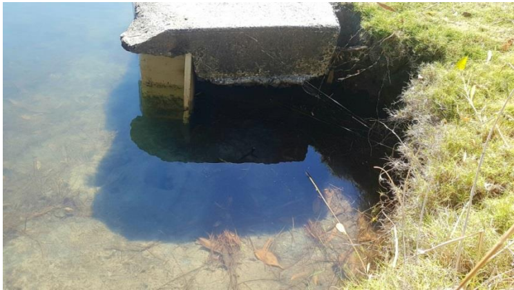
Figure 4: Extent of erosion – northern side
