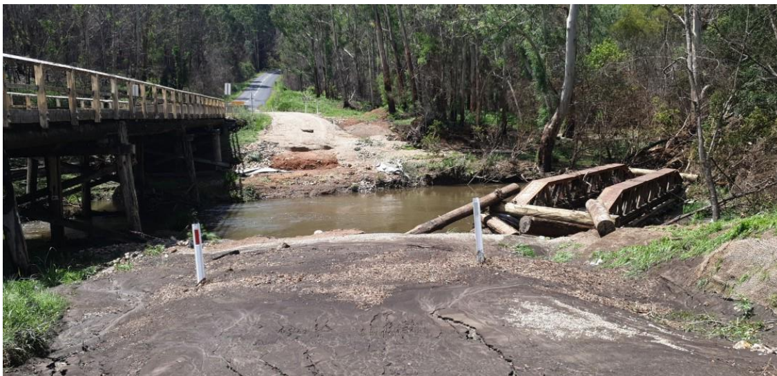
Figure 2 - Clouds Creek temporary bridge after being washed off its abutments
