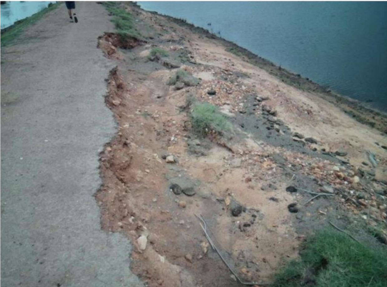
Figure 3 - Erosion Damage on The Avenue Levee (taken 10 th March 2020)
