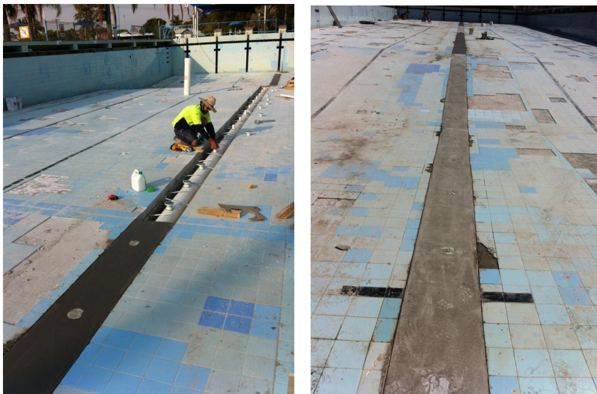
Figure 1 and 2 - Works completed in 2012 on the pool basin of the 50m pool
