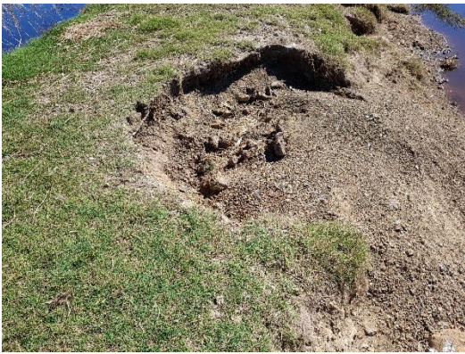
Figure 3: The Avenue Levee washout, Lavadia
