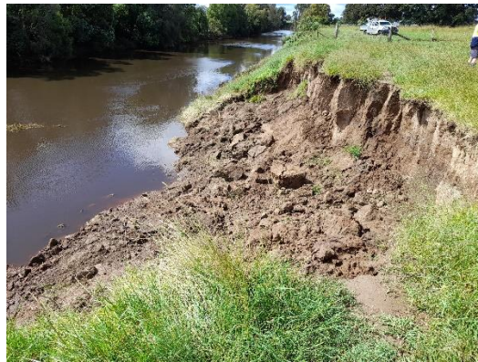
Figure 4: Swan Creek – Drain slumping
