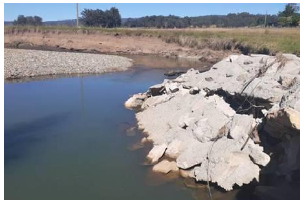
Figure 6: Tallawudja Creek Bridge (scour)
