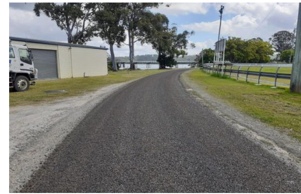
Item: Road - Fence - repair and replacement works Location: After - Riverfront area (outside)
