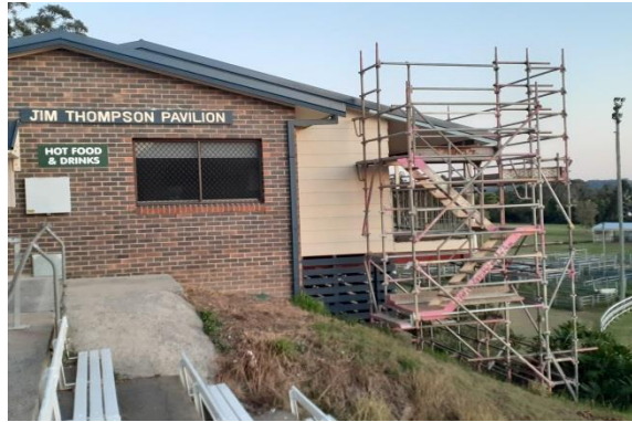
Item: JT Building - gas bottle relocate & new awning Location: Progress - existing uncovered veranda
