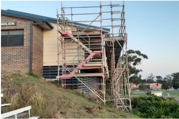
Item: JT Building - gas bottle relocate & new awning Location: Progress - existing uncovered veranda
