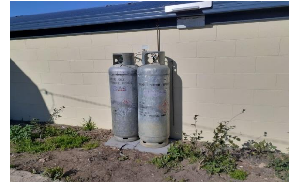
Item: JT Building - gas bottle relocate & new awning Location: After – relocated gas bottles
