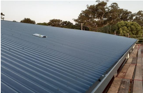
Item: JT Building - gas bottle relocate & new awning Location: After - covered veranda (roof)
