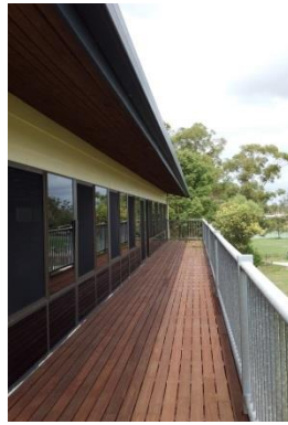
Item: JT Building - gas bottle relocate & new awning Location: Before - existing uncovered veranda
