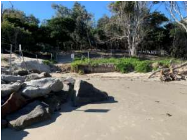
1 – End wall erosion at seawall impacting public access
