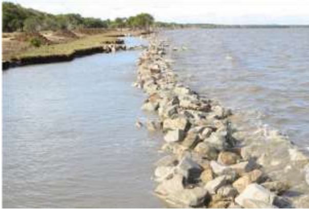
1 - rock fillets placed along a section of eroding shoreline, Wooloweyah Lagoon
