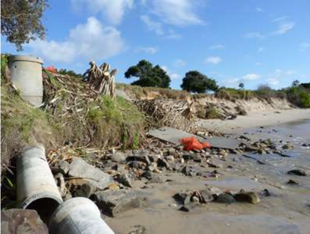
1 - Site after erosion event in 2012
