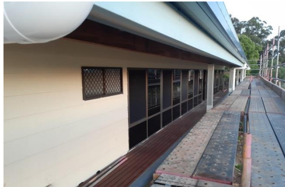
Item: JT Building - gas bottle relocate & new awning Location: After - covered veranda (deck & fascia)
