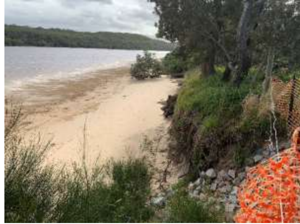
2 - erosion opposite Marine Rescue Tower threatening footpath
