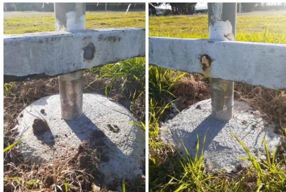
Item: Fence - repair and replacement works Location: After – concrete surround & new post base
