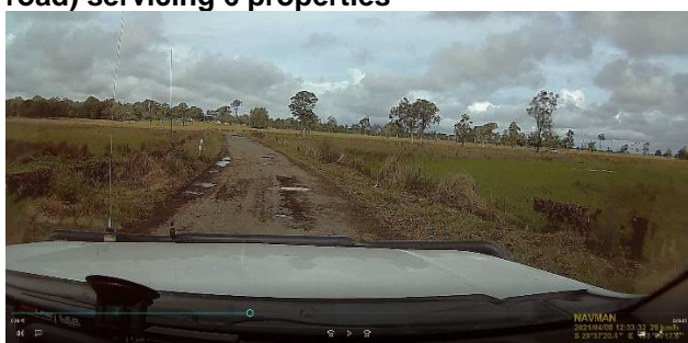
Figure 3: Gilletts Ridge Road damage caused by saturated pavement
