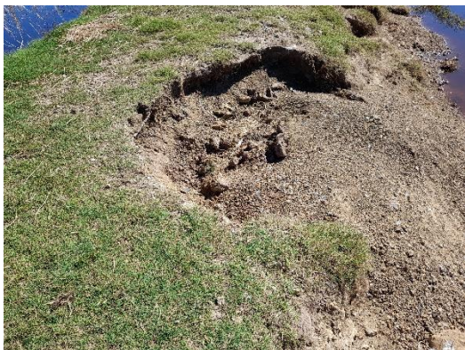
Figure 3: The Avenue Levee washout, Lavadia
