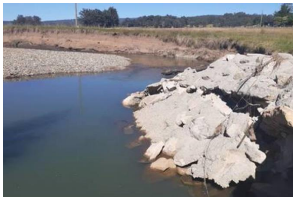
Figure 6: Tallawudja Creek Bridge (scour)
