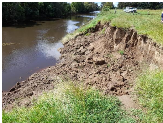
Figure 4: Swan Creek – Drain slumping
