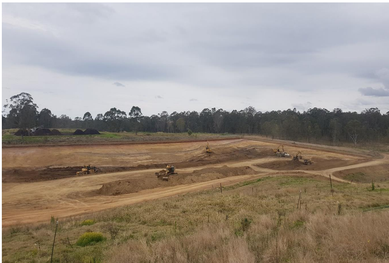
Plate 1 – View of active earthworks within the site of the new landfill cell. [Note: An area of unexpected rock strata is located towards the right end (as viewed in the above image) of the cell]
