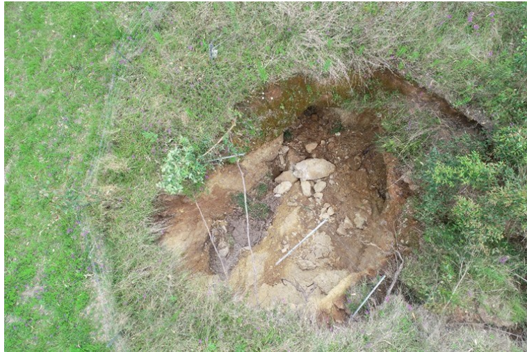
Sinkhole located over water supply tunnel which needs urgent repair.
