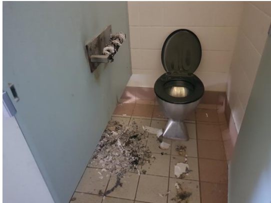
Public toilet vandalism, Market Square, Grafton
