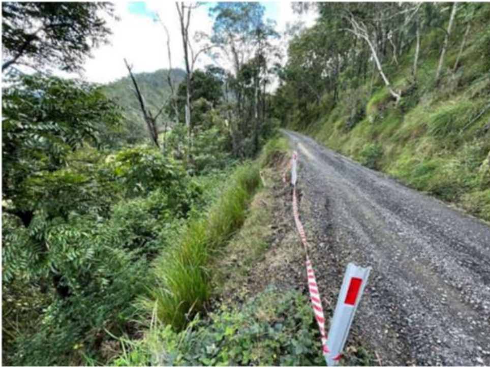
Figure 2: Major defect above. Landslip impacting travel lane, requires engineered solution for restoration.
