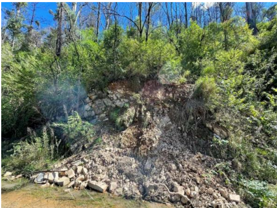
Figure 1: Minor defect above requiring upslope scaling and removal of loose material
