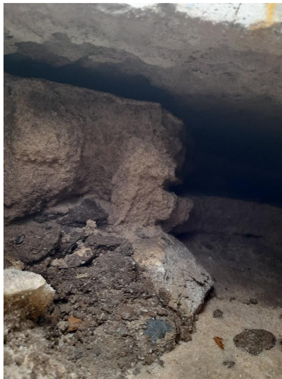
Extent of material loss (void) under the concourse slab
