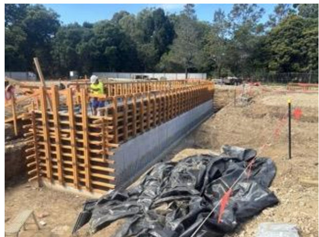
Figure 2: 25m pool balance tank
