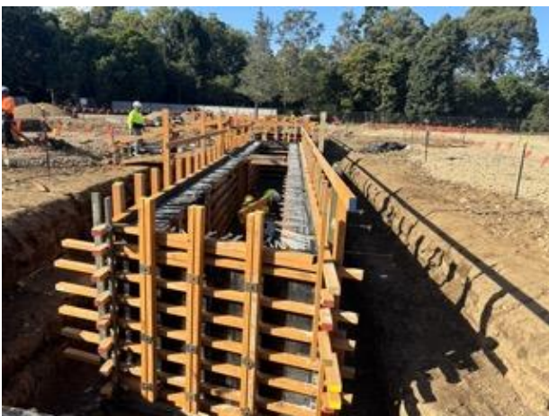
Figure 1: Leisure Pool balance tank
