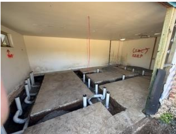
Figure 5: Sanitary drainage, front of house building
