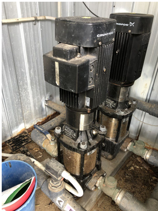
Figure 8. Irrigation pumps in irrigation shed. Note corrosion to the galvanised shed.
