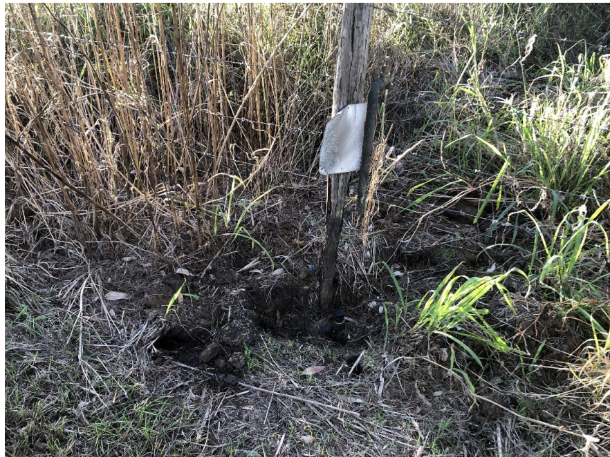
Figure 9. Damaged raiser that has been capped off. This raiser had been burnt and hidden in long grass, testing revealed this pipe is associated with the STP to wet weather dam pipeline. Many more like this have been located and capped.
