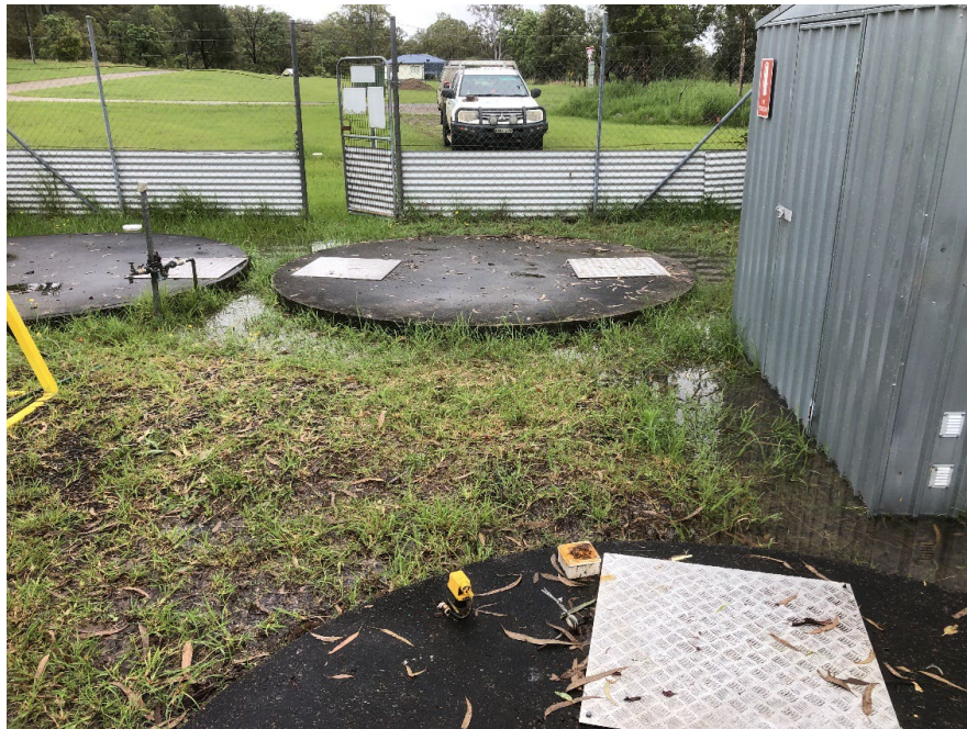
Figure 5. Main control shed flooding during major rain event.
