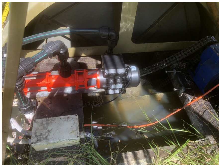
Figure 6. RBC flooded due to electrical issue resulting in high water levels.
