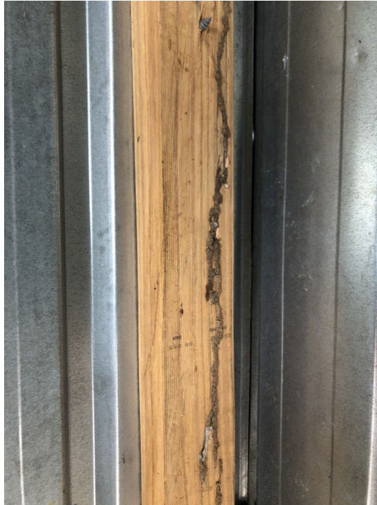
Figure 3. Termite damage within the main control shed.
