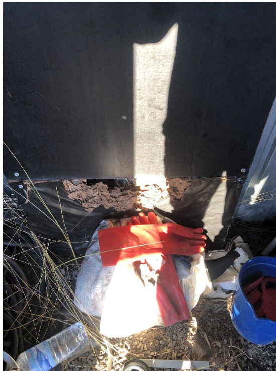
Figure 4. Termite damage and moisture rot damage within the main control shed.
