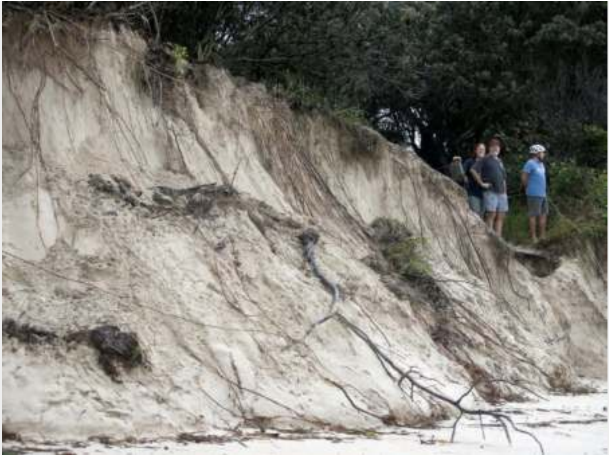
Byron Bay's erosion after wild weather and hazardous swells lash in 2020. Picture: Regi Varghese/Getty Images
